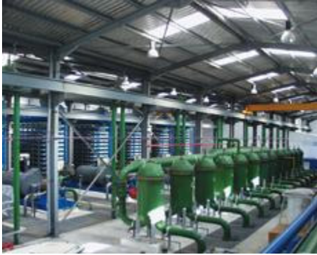
Plant view of the Caramondani Desalination Plants Ltd. facility in Dhekelia, Cyprus.
