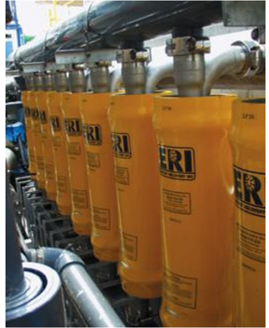
PX-220 large-rotor installation in Caramondani SWRO facility in Dhekelia, Cyprus
